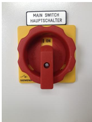
Picture 12. Main switch
