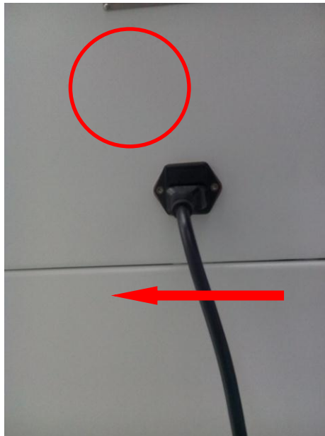
Picture 9. Power supply
