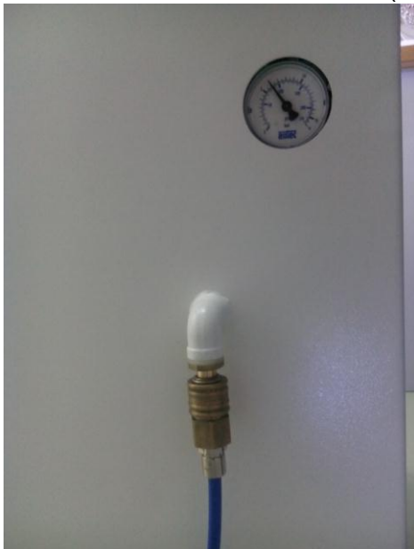
Picture 8. Compressed air connection
